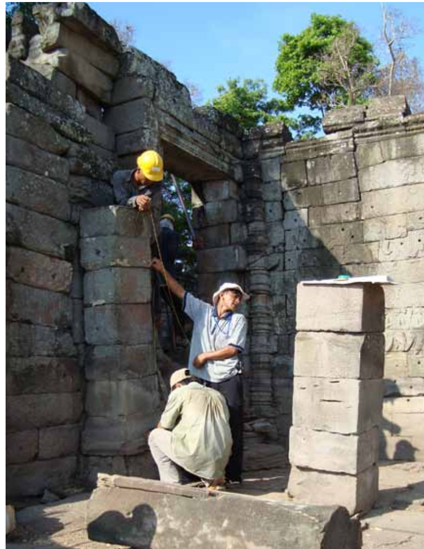
Above: Work continues on the Southeast sector of Bas Relief East Enclosure Wall Banteay Chhmar, Cambodia. © GHF
