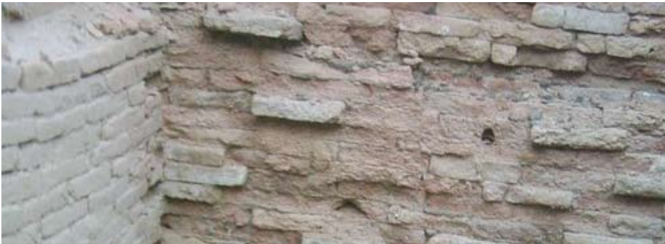
Soluble salt mobilization is a major conservation challenge at Ur, leading to the degradation of ancient bricks. Photo by © Global Heritage Fund
