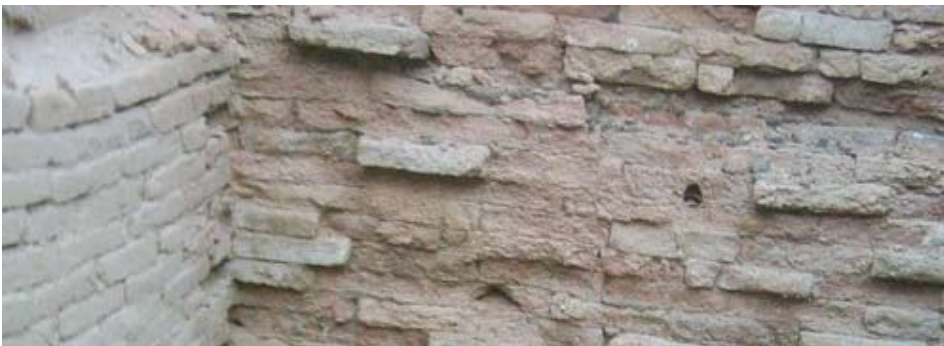
Soluble salt mobilization is a major conservation challenge at Ur, leading to the degradation of ancient bricks. Photo by © Global Heritage Fund
